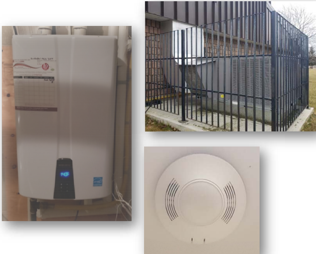
Figure 6: Photographs of the new high efficiency HVAC unit, instantaneous water heater and a motion sensor installed at the Community Centre.
