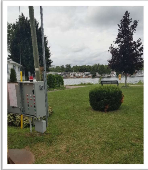
Fig 14 – SPS#1 - Grass field beside the pump control panel along Lakeshore Drive.
