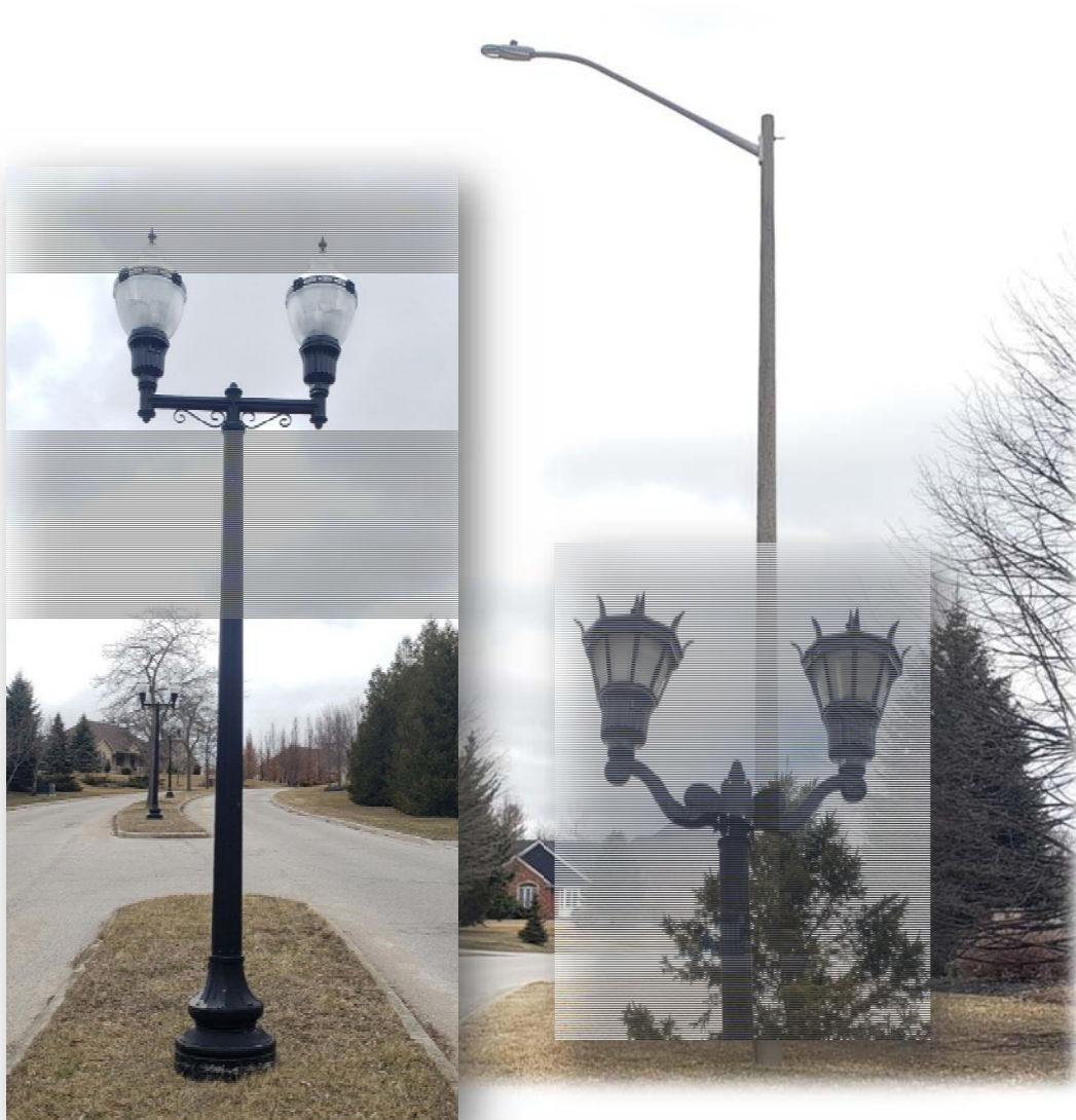
Figure 5: Photographs of the new LED outdoor street lighting
