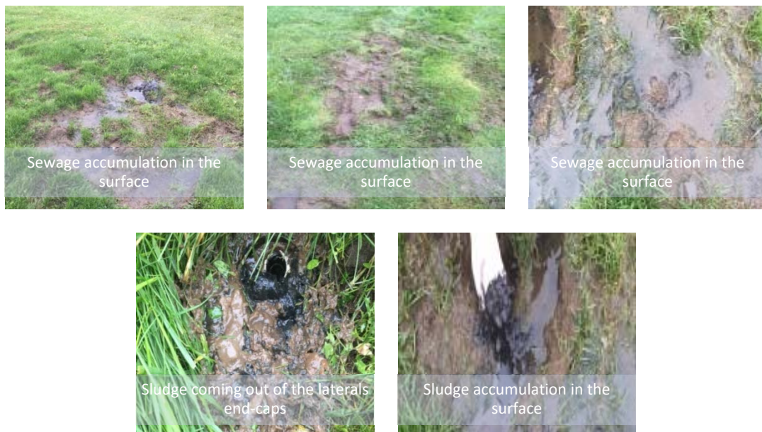
Figure 3-5: Sludge Deposition within the Subsurface Disposal System (Tile Beds)
