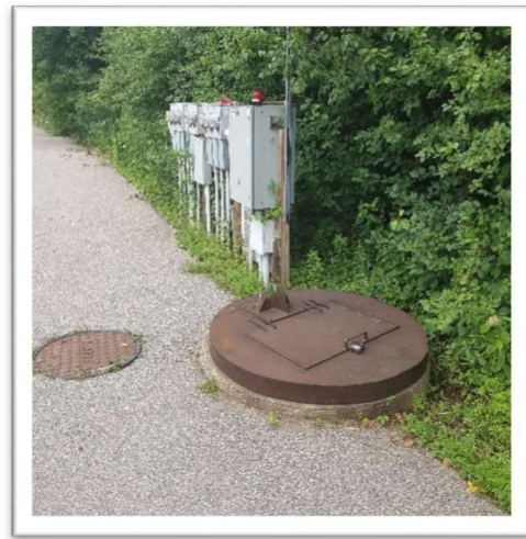
Fig 17 – SPS#5 – Green area beside the pump control panel. Landscaping needs to be done.
