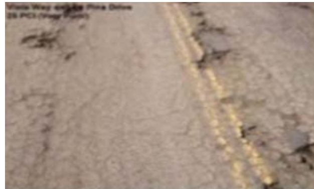
25 PCI (Very Poor)
